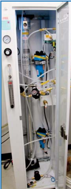
COMMERCIAL AIR NITROGEN SYSTEM
