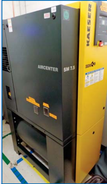
PURCHASED/ INSTALLED 2014 KAESER AIRCENTER AIR COMPRESSOR
