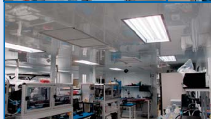
MECART CLEAN ROOM
